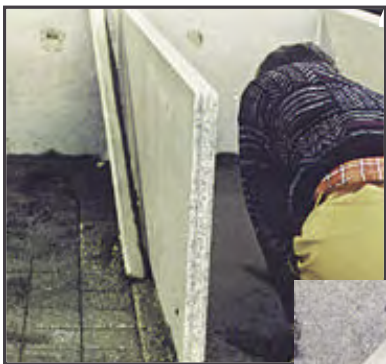
12. A craftsman pours each side of the floor to a thickness of 6".
