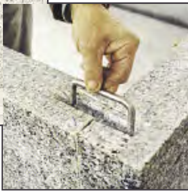
11. A stainless steel c-clamp is used to join the back and side walls.
